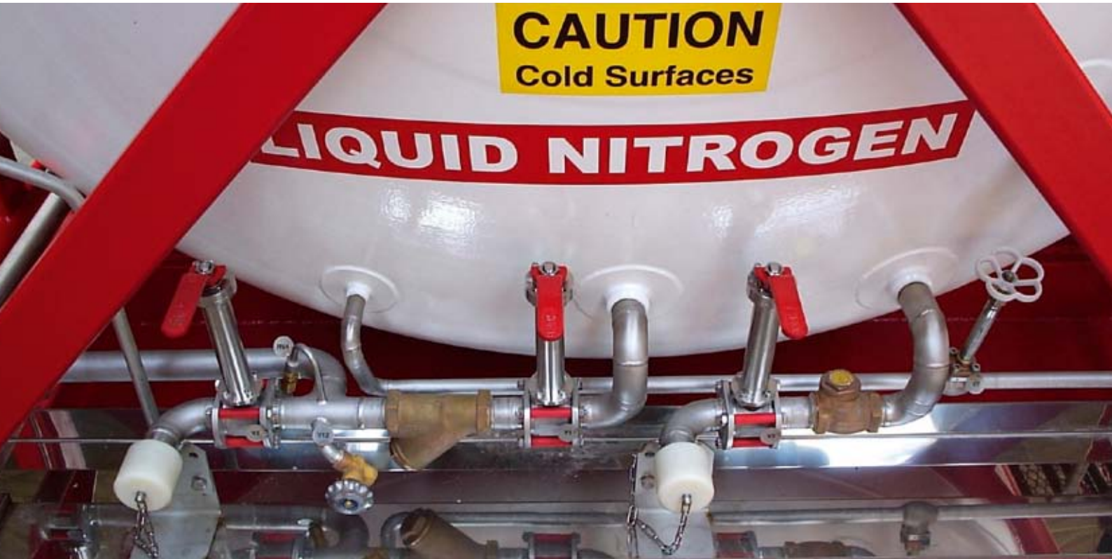
Cryogenic valves on mobile tank
