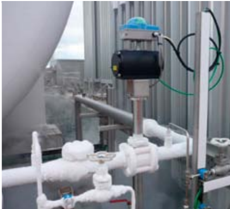
Cryogenic valve at the outlet of a liquid nitrogen tank
