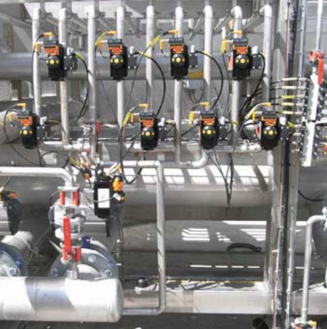
Valves with actuators on agrochemical process
