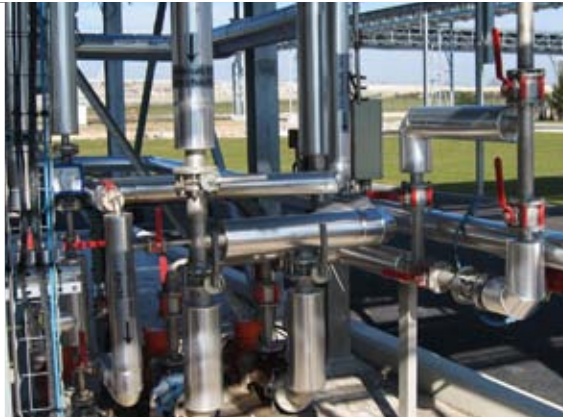
Installation in bio-fuel refinery
